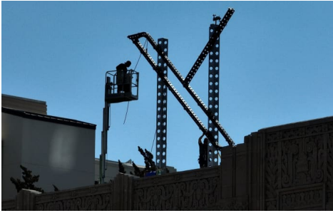
Workers dismantled a new X logo on the roof of the headquarters on July 31, after the city launched an investigation into its installation. PHOTO: JUSTIN SULLIVAN/GETTY IMAGES
